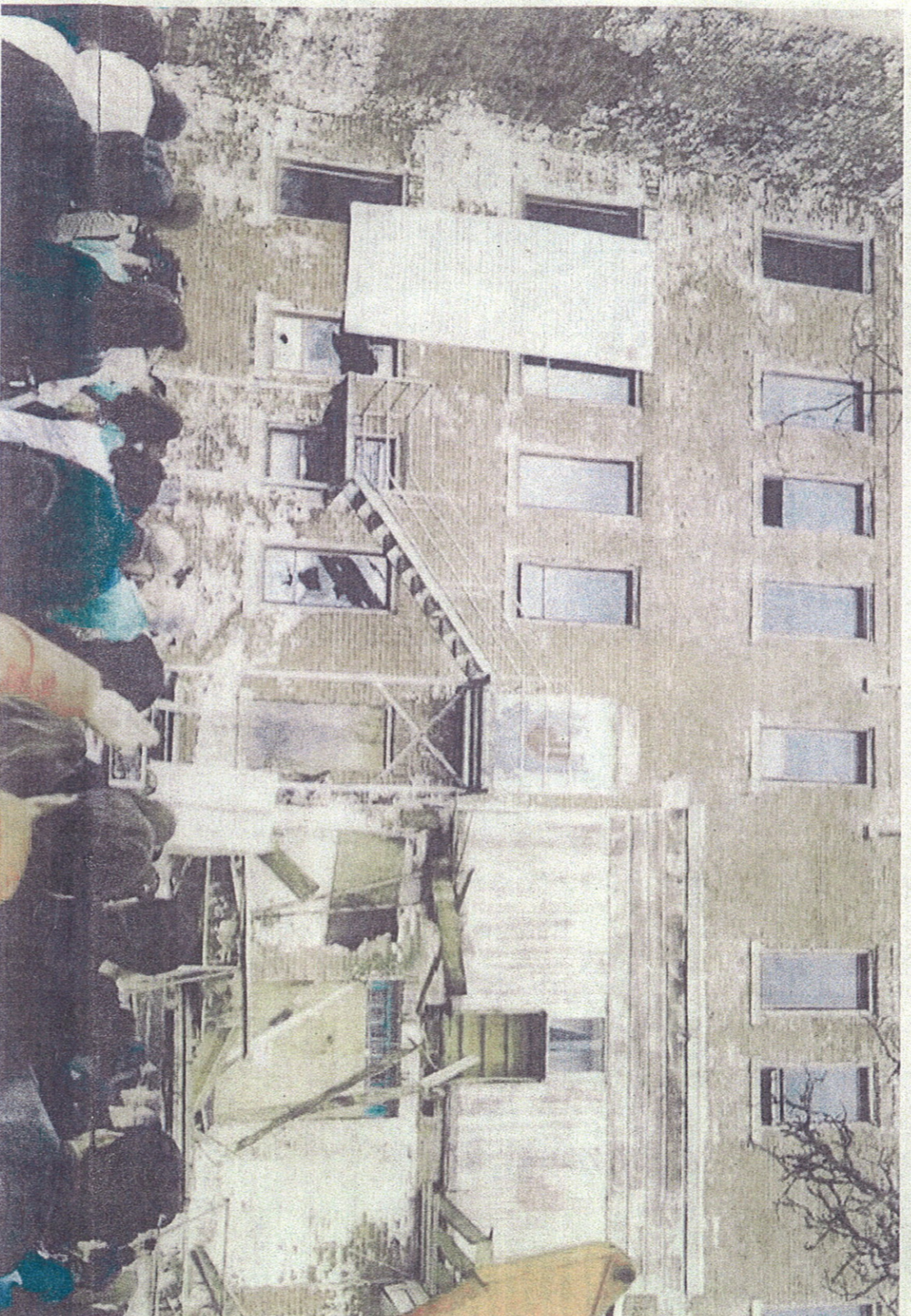
CHIEF BOB CHAMBERLAIN A crowd in Alert Bay watches the demolition of St. Michael's Indian Residential School on Wednesday. The school operated from 1929 to 1974.
